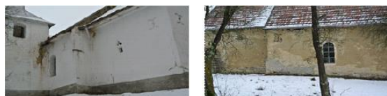
Fig.6. Degradation of northern and southern facade
