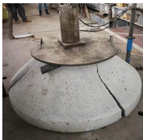
Fig. 6. Manhole element with DN160, after cracking, at failure
