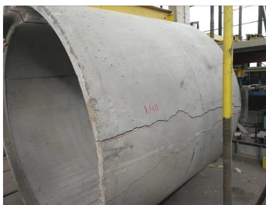
Fig. 4. Manhole straight element with DN200, after cracking, at failure
