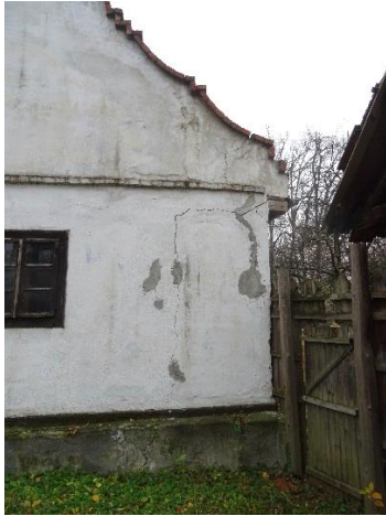
Fig. 37. Cracks on the exterior of the house
