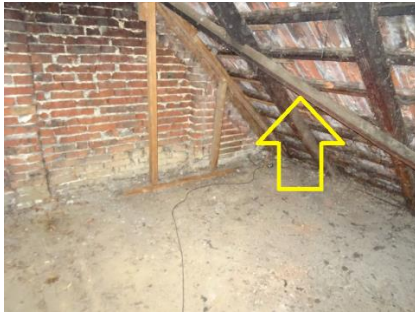
Fig. 10. Stiffeners for the roof
