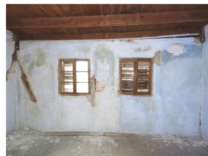
Fig. 36. Masonry infill separation cracks visible inside the house
