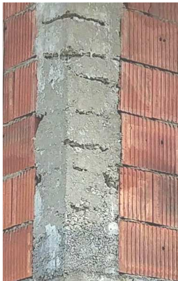
Fig. 2. Segregation of concrete in a corner column of a confined masonry structure
