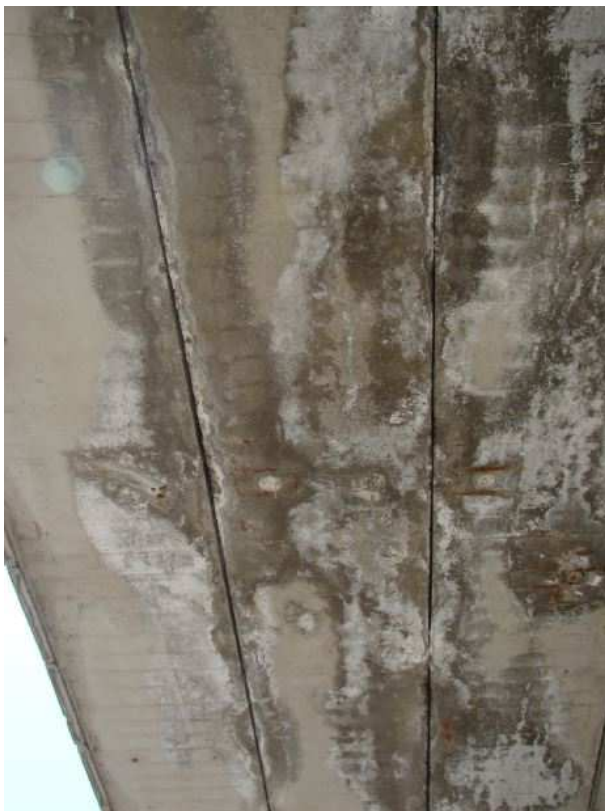
Fig. 6. Marginal deteriorated beams
