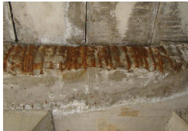
Fig. 7. Corrosion of reinforcement
