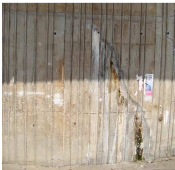
Fig. 3. Crack in the retaining walls
