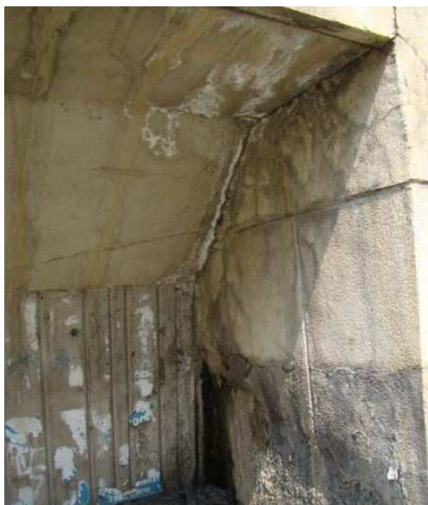
Fig. 4. Degradation of the retaining walls
