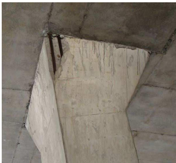
Fig. 9. Exfoliation of the new concrete layer
