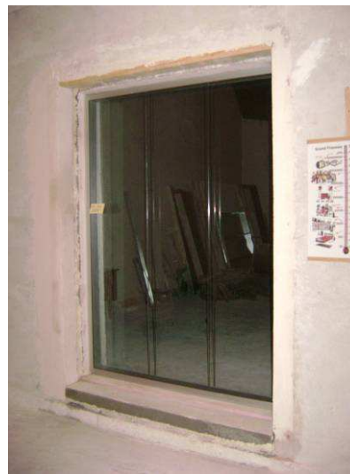
Fig. 1. Detail of the positioning of the VITRUM type (10 safety glass-73-10 safety glass) partition wall system in the airborne sound insulation stand
