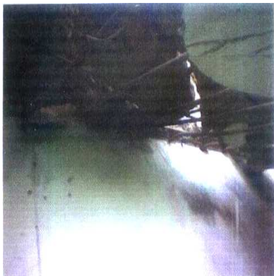
Fig. 2. Damaged floor slab with exposed reinforcement
