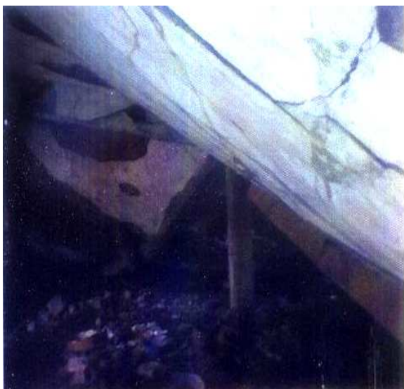
Fig. 1. Building section showing collapsed column, slab and beam
