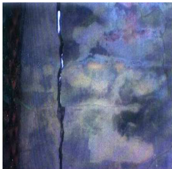
Fig. 3. Crack in the wall close to a column
