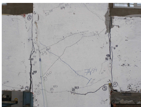
Fig. 4. Damage concentration at column-beam interface
