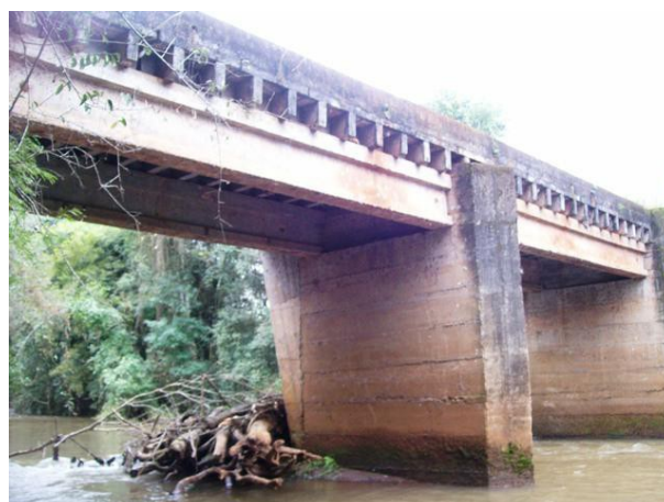
Figure 13. Tree trunks impacting on the pillar
