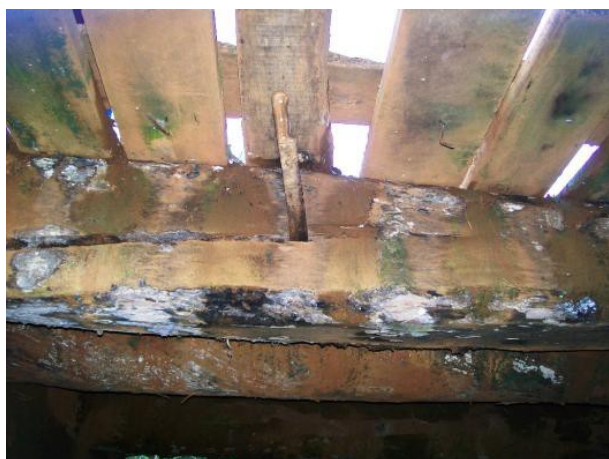
Figure 23. Disruption of the beam and fungi attack
