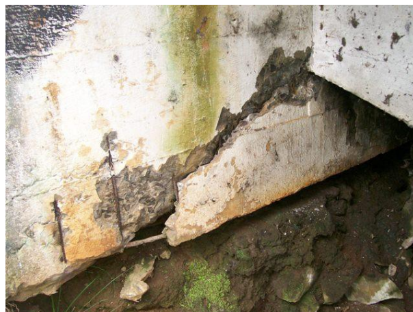
Figure 12. Disruption of the access balance of the bridge structure
