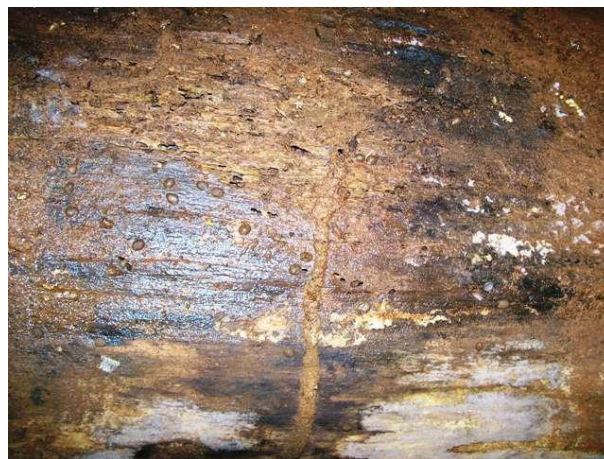
Figure 17. Insect attack in logs (beams) of the bridge support
