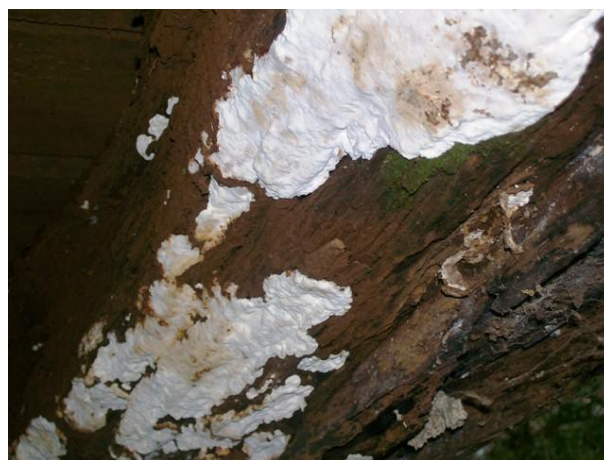
Figure 16. Wood attack by bacteria and fungi (Bridge P119)
