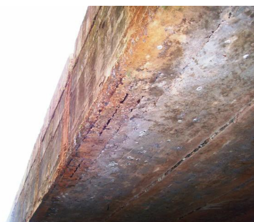
Figure 9. Reinforcement corrosion of the side beam of the bridge
