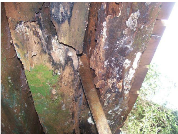
Figure 19. Wooden beam at an advanced stage of decomposition
