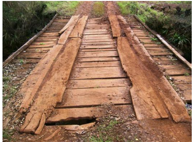
Figure 20. View of the board showing extensive damage
