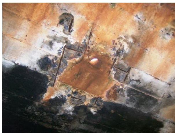
Figure 8. Peeling of concrete and corrosion of reinforcement
