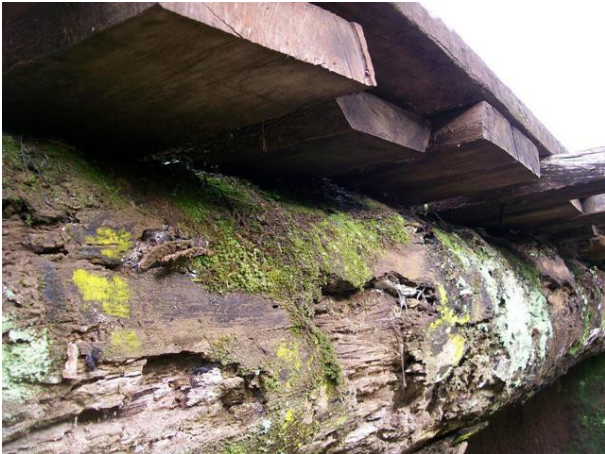
Figure 18. Bridge beam rotting
