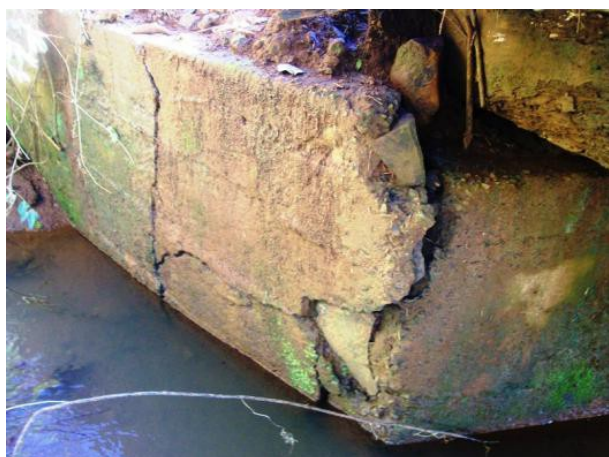
Figure 14. Disruption of the support and containment concrete of the bridge
